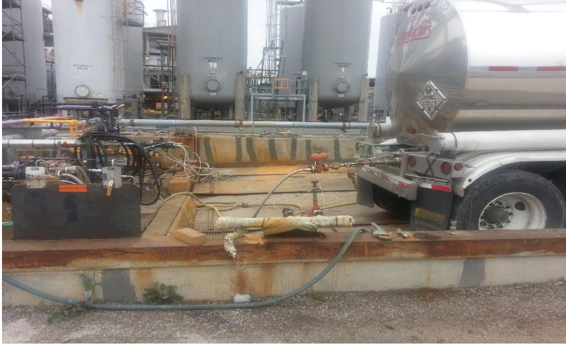
Figure 11 Tanker at Incinerator
