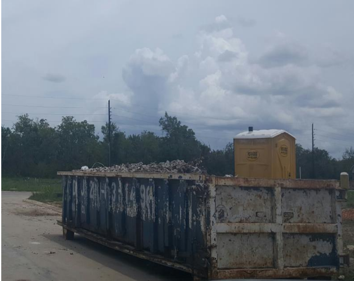
Figure 14 Waste Container Filled with Construction Debris
